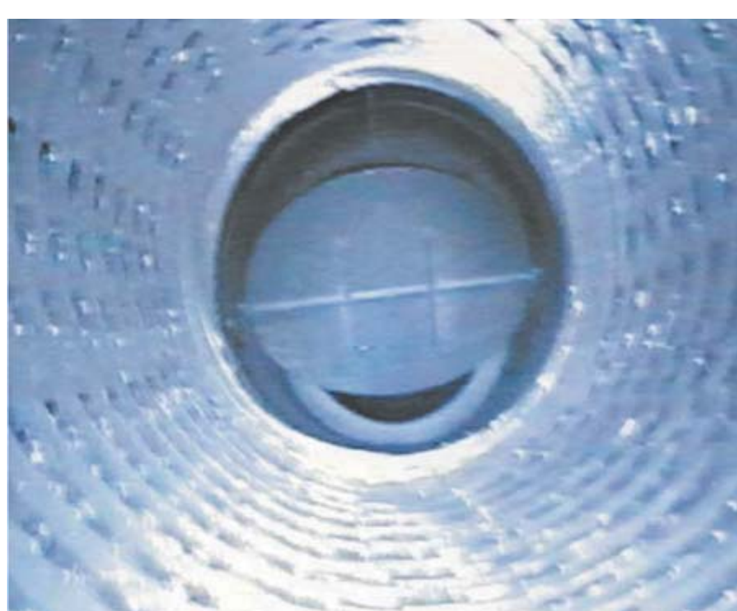
Air duct after cleaning.
