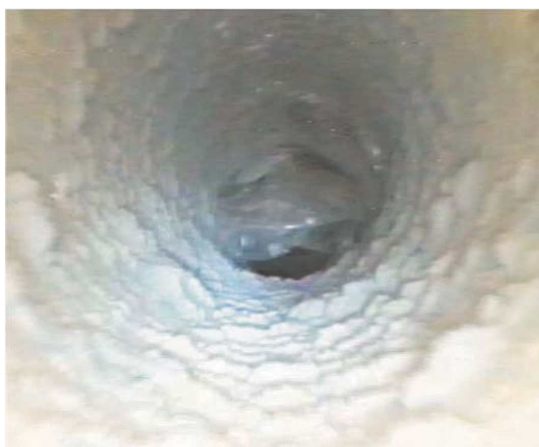
Dirty supply air duct in a hospital.
